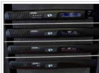
MX Control units
